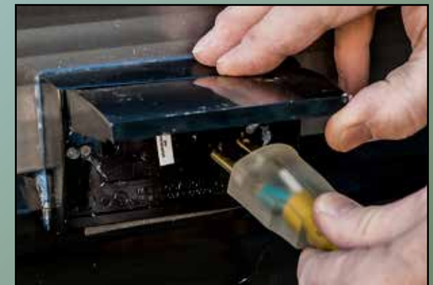
Convenient Outside GFCI Protected and Covered Outlet.
