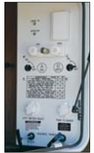
New Style Utility Center
