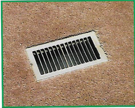
▲ Floor-ducted heat system provides balanced heat distribution. The duct system itself is sealed and insulated to avoid an inefficient loss of heat.
